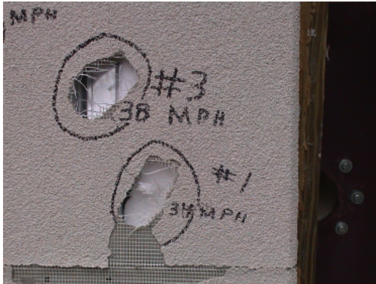
Figure 2. Photograph Showing Typical Missile Damage to Textured Surface Layer
